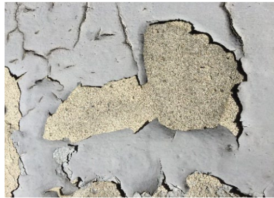
Figure 5. Peeling lead paint
